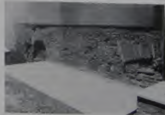
Fig. 75. S. Maria. East part of aisle wall. Brick construction, masonry, cornice, ledges, masonry, Roman construction.
